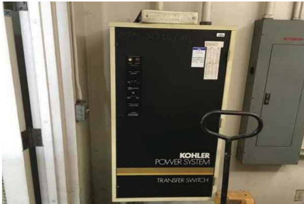
33 AUTOMATIC TRANSFER SWITCH
