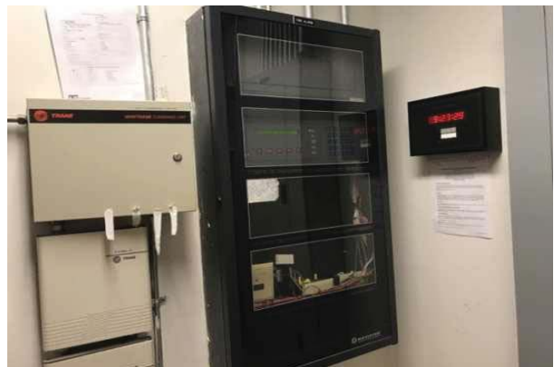
42 FIRE ALARM CONTROL PANEL
