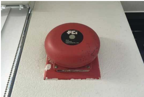
35 OUTDATED FIRE ALARM SYSTEM
