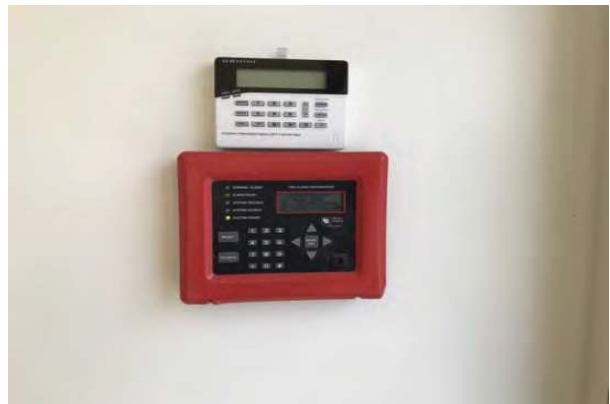
46 ANNUNCIATION ALARM PANEL
