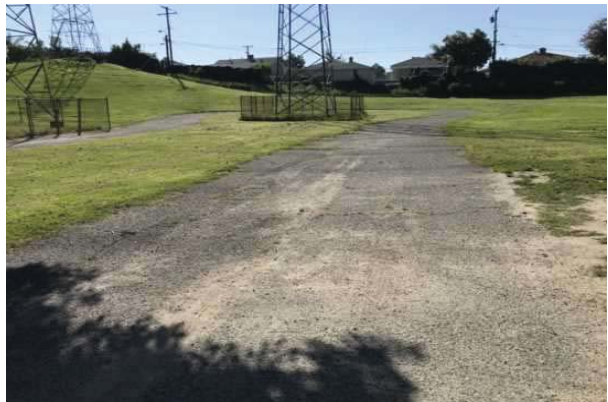
12 POOR ASPHALT PAVEMENT DRIVEWAY
