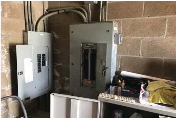
45 POOL HOUSE DISTRIBUTION PANEL
