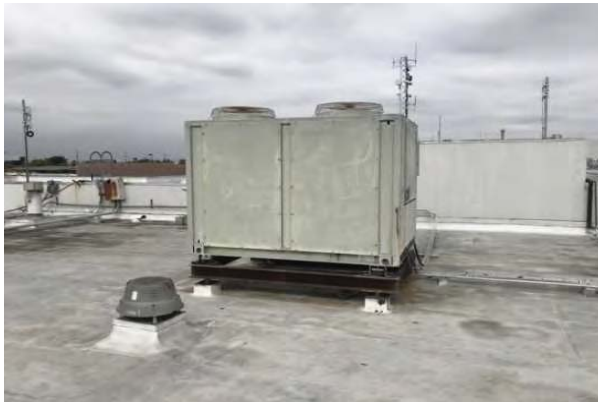
33 CONDENSING UNIT\REMOTE CHILLER
