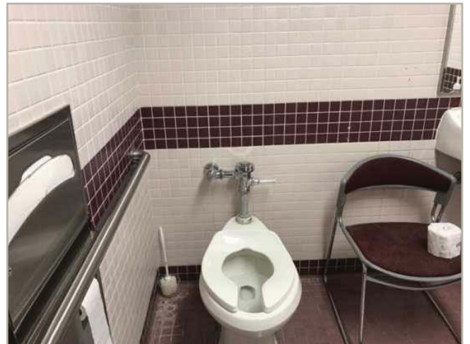
Missing grab bar
