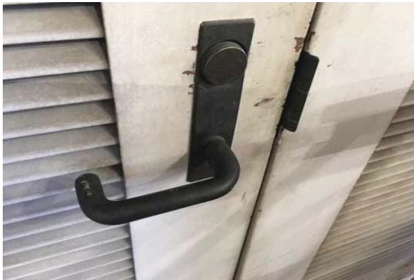
21 FAULTY INTERIOR DOOR HARDWARE
