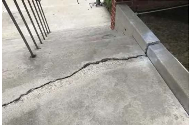
8 STRUCTURAL CONCRETE MOVEMENT
