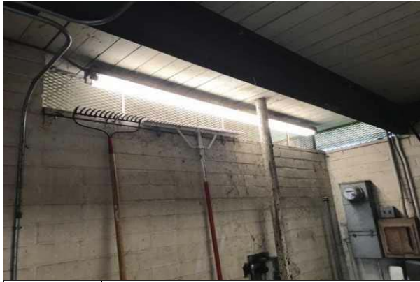
43 INTERIOR LIGHTING SYSTEM
