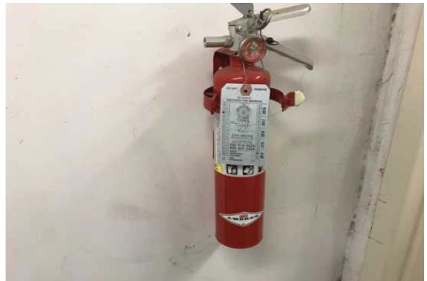
54 COMMUNITY CENTER FIRE EXTINGUISHER
