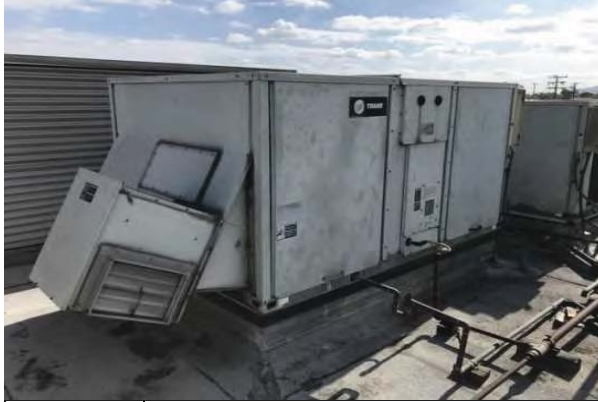
31 PACKAGED UNIT (RTU)
