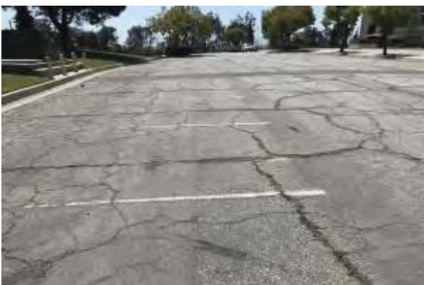
5 DETERIORATED PARKING LOTS
