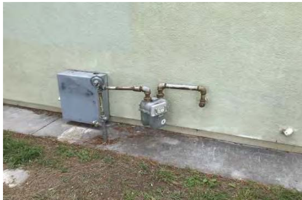
60 COMMUNITY CENTER GAS METER
