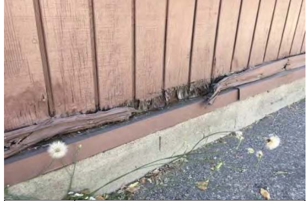
14 DETERIORATING WOOD SIDING
