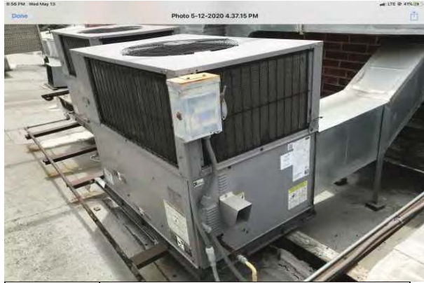
26 PACKAGED UNIT (RTU)
