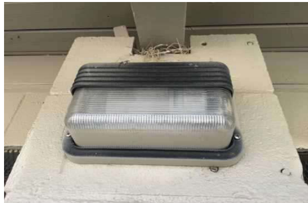
18 EXTERIOR BUILDING MOUNTED LIGHT
