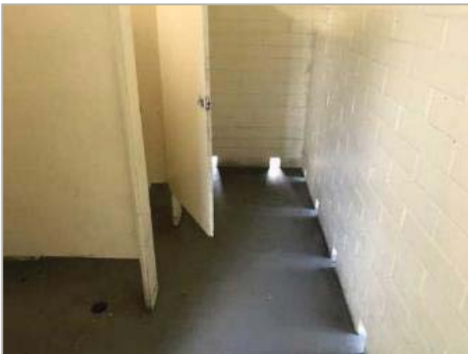
Lack of Accessible restroom
