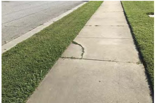
10 DAMAGED PEDESTRIAN PAVEMENT SIDEWALK
