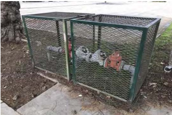
23 SITE - BACKFLOW PREVENTER
