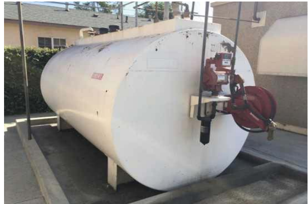
28 FUEL STORAGE TANK
