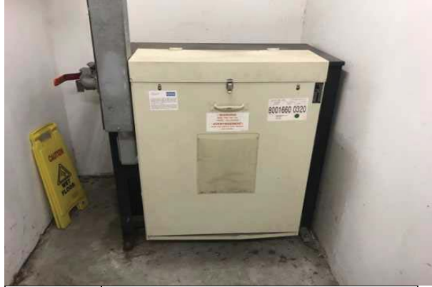
56 COMMUNITY CENTER ELEVATOR, HYDRAULIC
