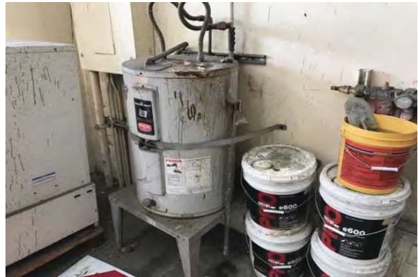
40 WAREHOUSE WATER HEATER
