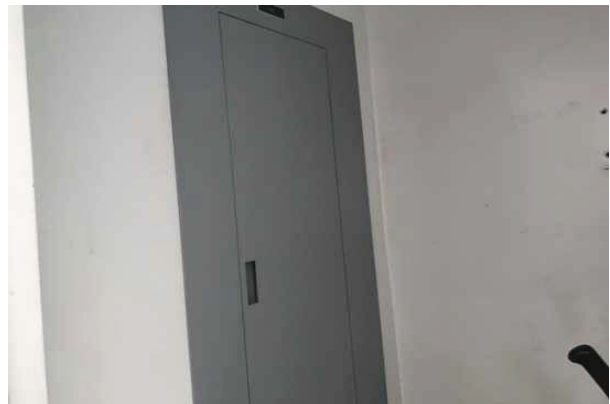
40 DISTRIBUTION ELECTRICAL PANEL
