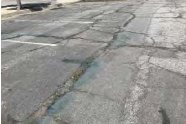
7 DETERIORATED PARKING LOTS
