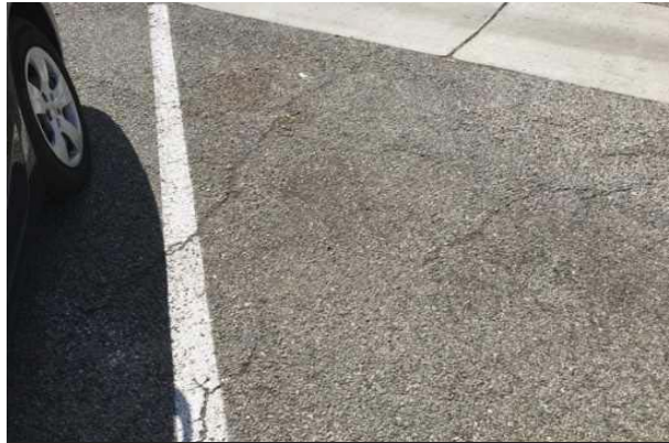
8 ALLIGATOR CRACKING IN PARKING ASPHALT
