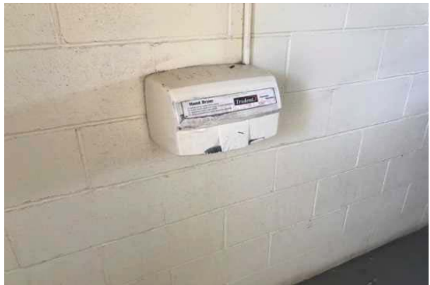
48 RESTROOM HAND DRYER
