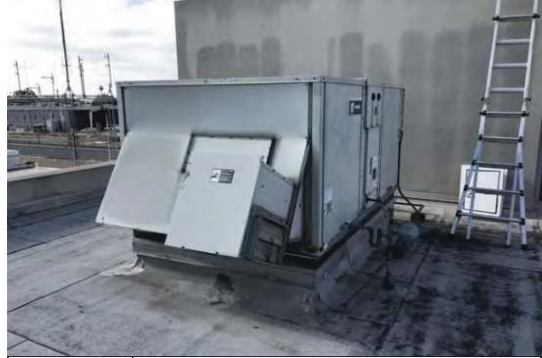
32 PACKAGED UNIT (RTU)
