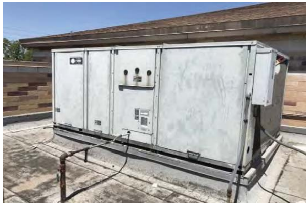
36 YOUTH CENTER PACKAGED UNIT (RTU)
