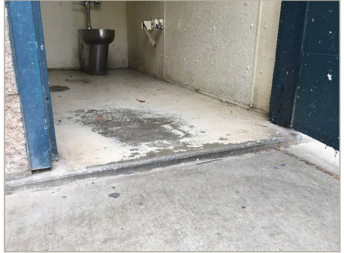
Inaccessible building entrance at playground restroom
