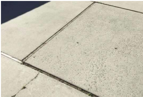
29 MISSING JOINT CAULKING IN CONCRETE PAVEMENT
