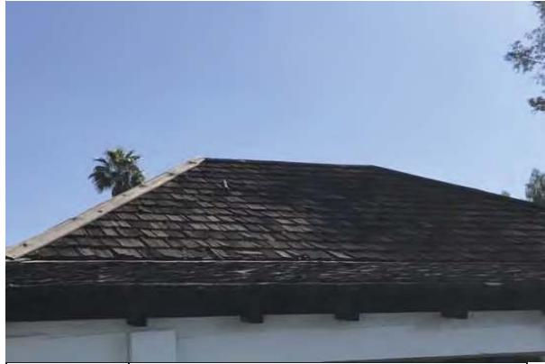
32 DAMAGED ROOF AREAS
