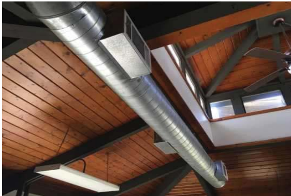
15 HVAC SYSTEM DUCTWORK
