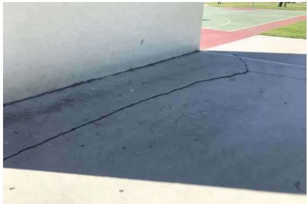
30 CRACKED PEDESTRIAN PAVEMENT SIDEWALK
