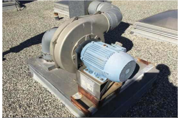
26 ROOF MOUNTED VEHICLE EXHAUST FAN
