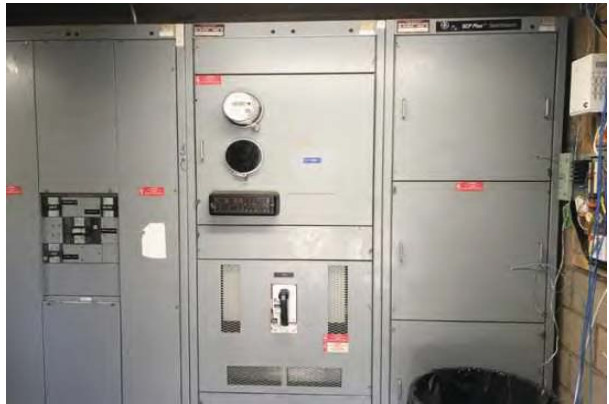
10 SENIOR CENTER SWITCHBOARD
