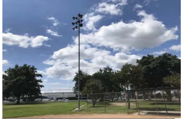
20 SOFTBALL FIELD POLE LIGHT
