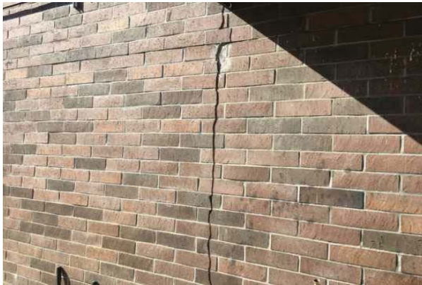
15 CRACKED BRICK VENEER FAÇADE
