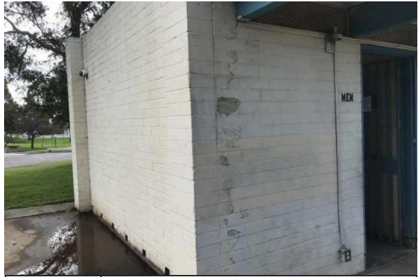
32 DETERIORATED EXTERIOR WALLS
