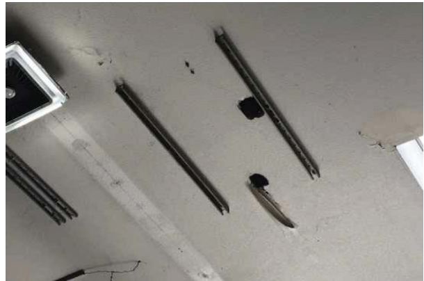
22 HOLES IN GYPSUM BOARD CEILING
