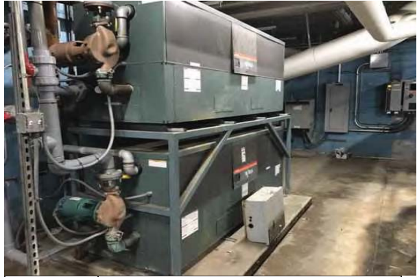
20 CITY POOL BUILDING - POOL HEATERS
