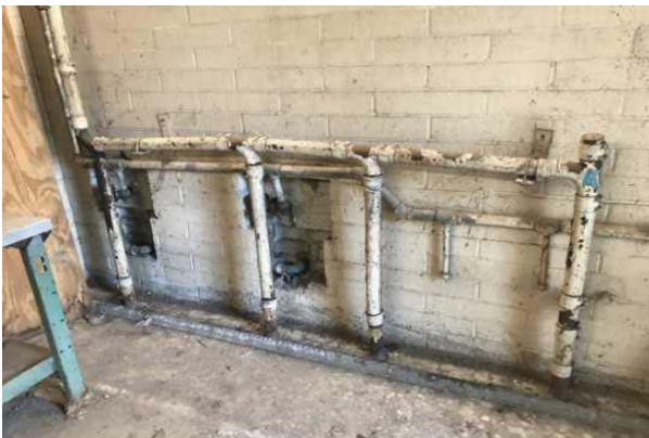
41 RESTROOM PLUMBING SYSTEM
