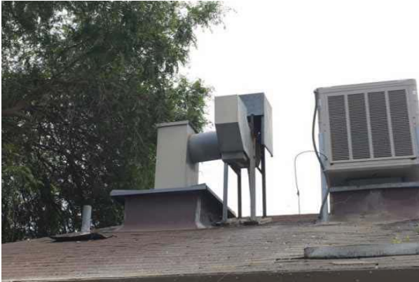
21 ROOF MOUNTED EXHAUST FAN
