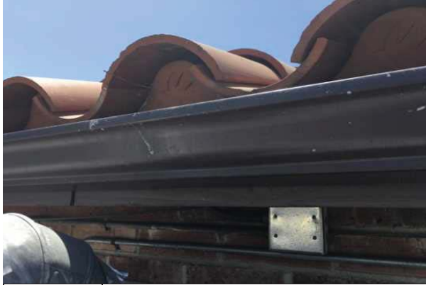
19 BIRDS NESTING IN BETWEEN THE ROOF TILES
