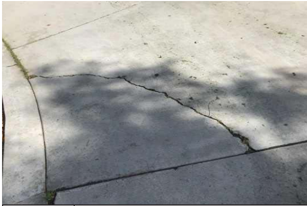
19 CRACKED PEDESTRIAN SIDEWALK
