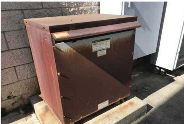
39 CORRODED SECONDARY TRANSFORMER
