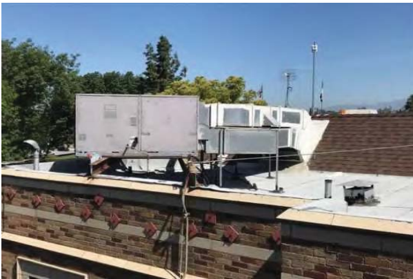
11 SENIOR CENTER PACKAGE UNIT (RTU)
