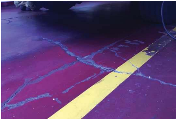
21 CRACKED CONCRETE FLOORING
