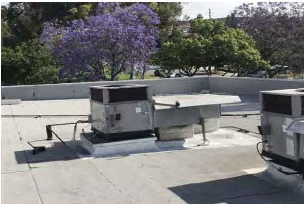
21 PACKAGED UNIT (RTU)
