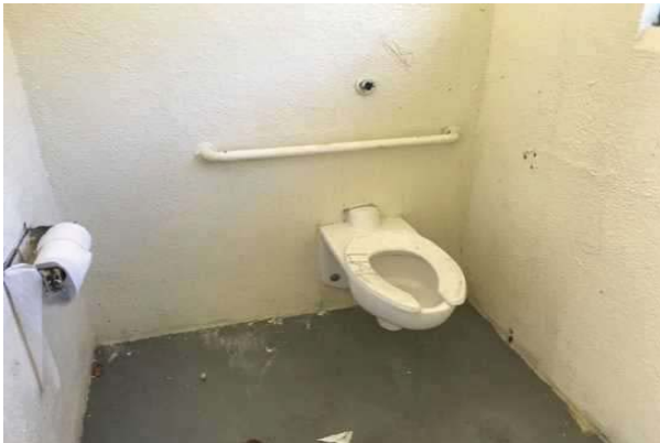
45 MISSING ADA TOILET GRAB BAR
