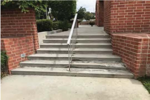
7 DAMAGED EXTERIOR STAIRS
