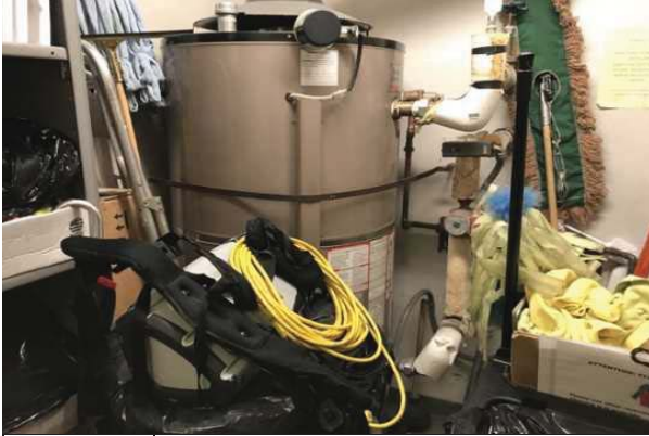
37 ADMINISTRATION OFFICE BUILDING WATER HEATER
