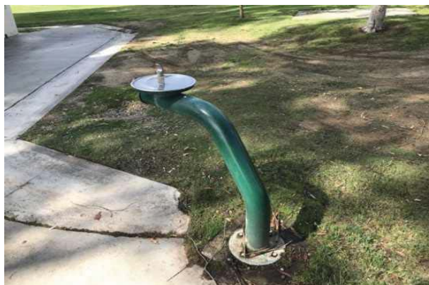
12 FLOODED DRINKING FOUNTAIN
