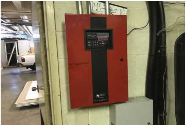
45 FIRE ALARM PANEL
