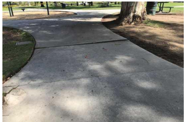
18 UNEVEN PEDESTRIAN SIDEWALK
