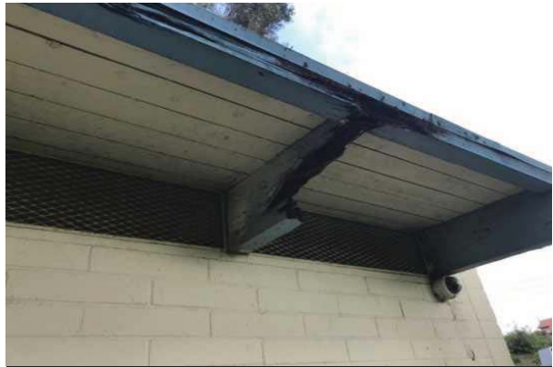
34 DETERIORATED ROOF STRUCTURE
