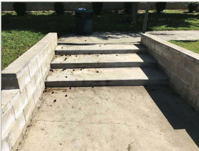
Inaccessible site stairs to main park area
