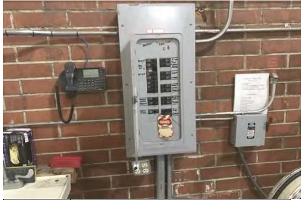
32 ELECTRICAL DISTRIBUTION PANEL
