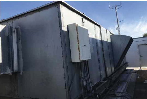
27 EXTERIOR AIR HANDLER (AHU)
