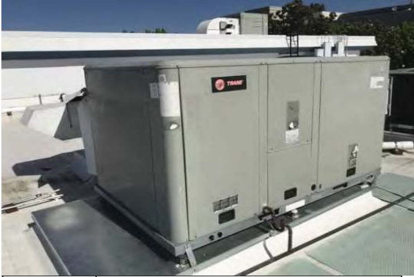
37 PACKAGED UNIT (RTU)
