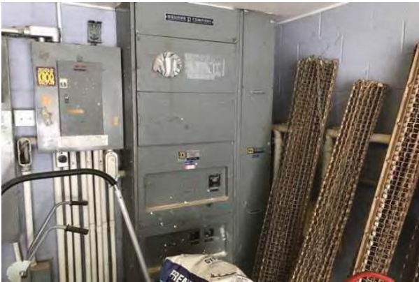
51 RESTROOM BUILDING SWITCHBOARD
