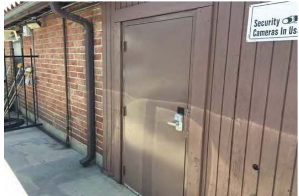
16 EXTERIOR STEEL DOOR
