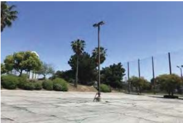
11 PARKING POLE LIGHT
