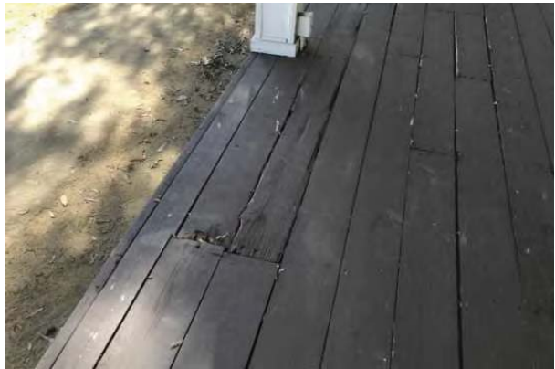
22 DAMAGED WOOD FLOORING
