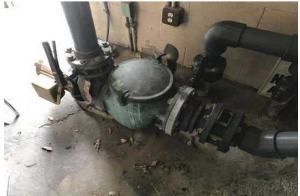
46 SWIMMING POOL CIRCULATION PUMP
