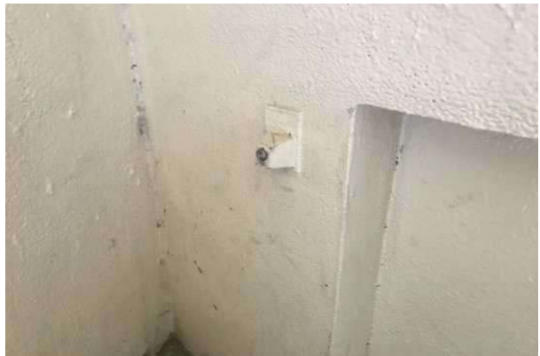
48 NON-OPERATIONAL HAND DRYER
