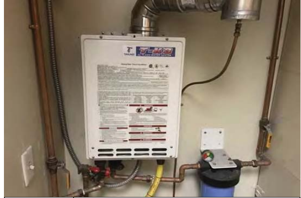
38 SHOP- INSTANT WATER HEATER
