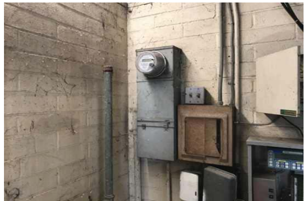
42 ELECTRICAL SYSTEM DISTRIBUTION PANEL
