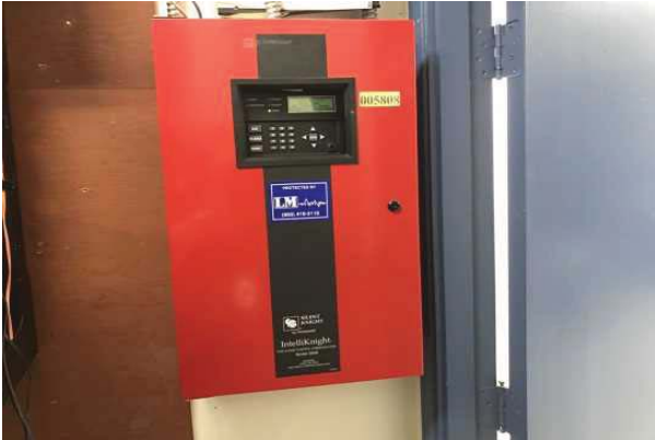
25 FIRE ALARM CONTROL PANEL
