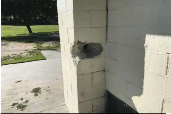
7 DAMAGED CMU EXTERIOR WALL
