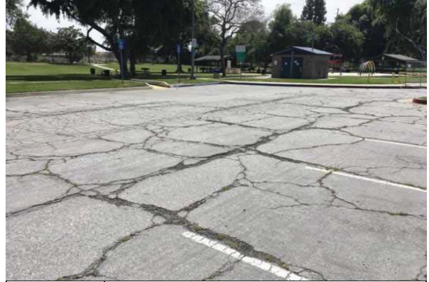
38 CRACKED ASPHALT PAVEMENT
