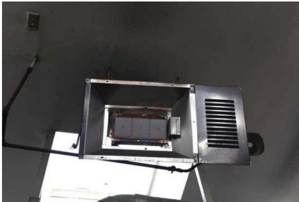
27 SUSPENDED UNIT HEATER
