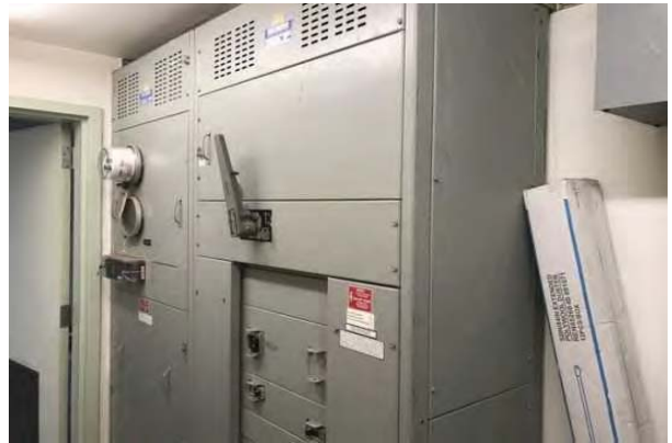
52 COMMUNITY CENTER BUILDING SWITCHBOARD
