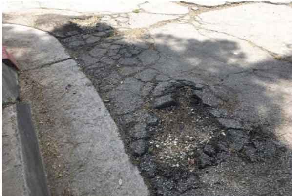
39 ASPHALT PAVEMENT POTHOLE
