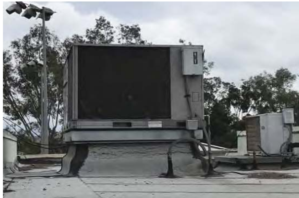
58 COMMUNITY CENTER RTU
