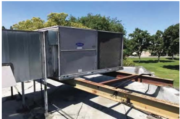
12 SENIOR CENTER PACKAGE UNIT (RTU)
