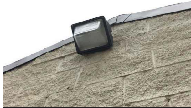
32 EXTERIOR BUILDING MOUNTED LIGHT
