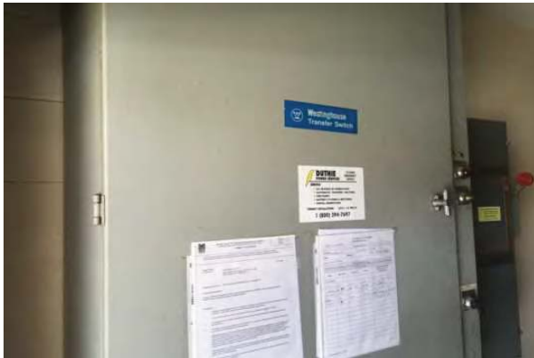
27 AUTOMATIC TRANSFER SWITCH
