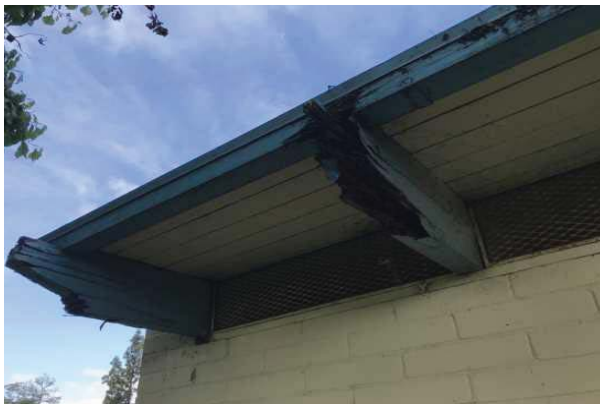
35 DETERIORATED ROOF STRUCTURE
