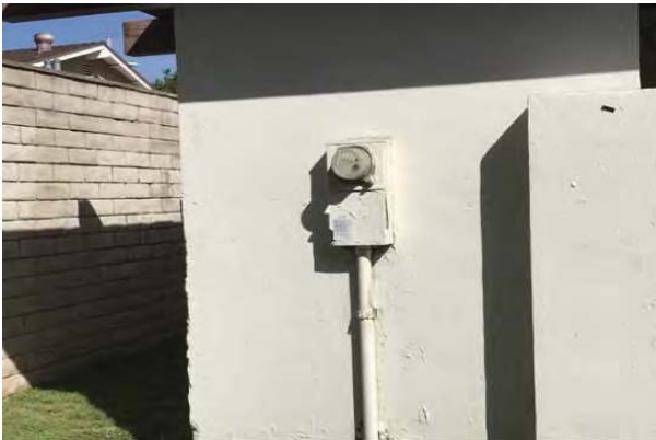
39 ELECTRICAL DISTRIBUTION SYSTEM
