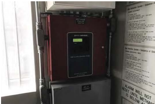
45 FIRE ALARM CONTROL PANEL
