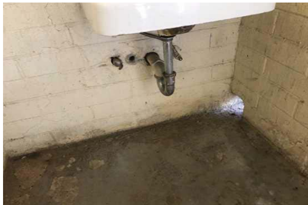
48 MISSING LAVATORY ADA PIPE WRAPS
