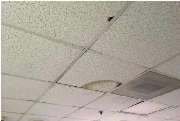
23 STAINED, WORN, AND BROKEN ACT
