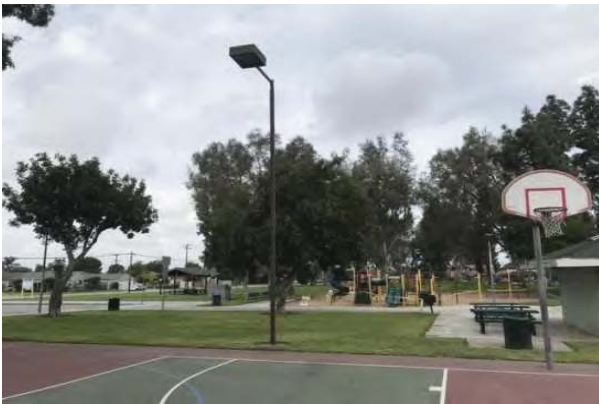
23 BASKETBALL COURT LIGHT POLE
