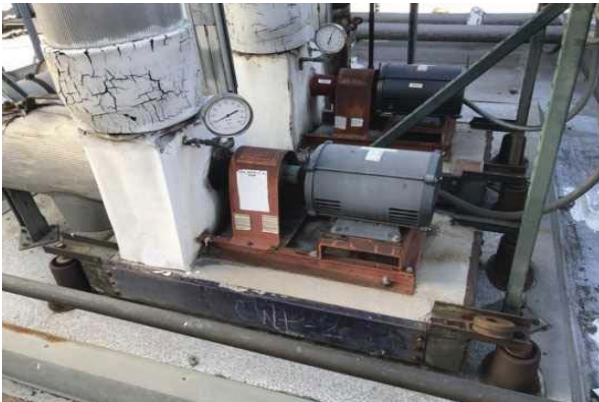
33 DOMESTIC CIRCULATION/BOOSTER PUMP
