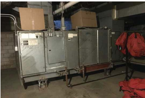
29 INTERIOR AIR HANDLER (AHU)
