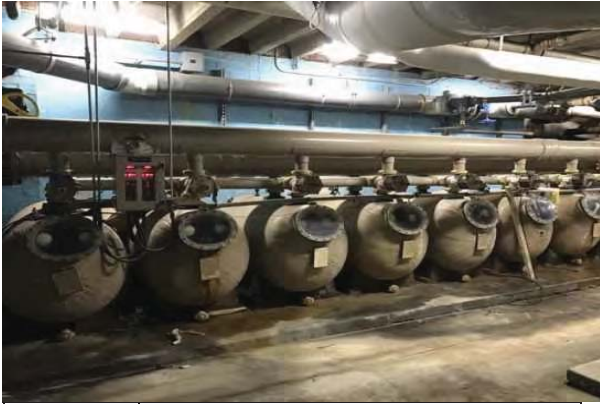
19 CITY POOL BUILDING - POOL FILTRATION SYSTEM
