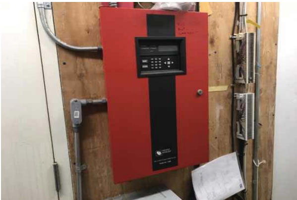
53 COMMUNITY CENTER FIRE ALARM PANEL
