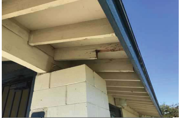
8 DAMAGED ROOF STRUCTURE
