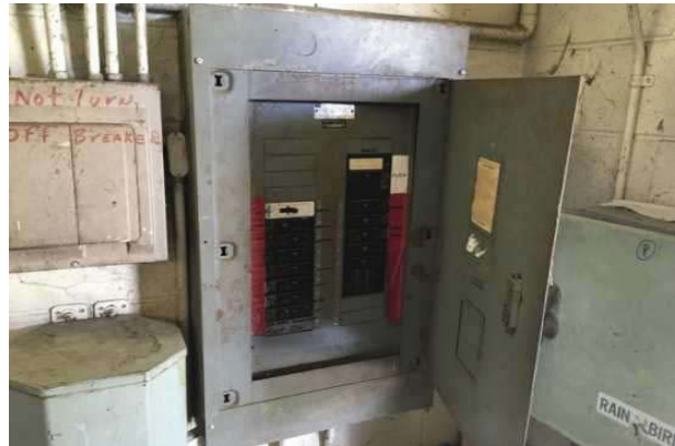
16 MAIN DISTRIBUTION PANEL
