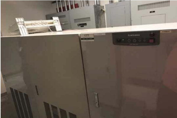
37 UNINTERRUPTIBLE POWER SUPPLY (UPS)
