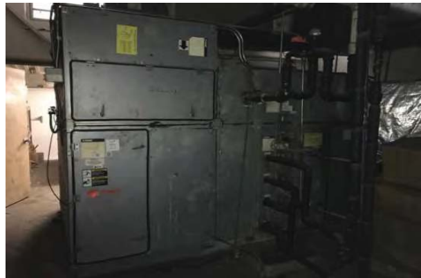
36 AIR HANDLER (AHU) - (BUILDING 311)
