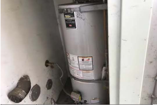
55 COMMUNITY CENTER WATER HEATER
