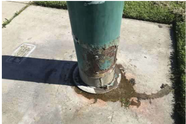
28 DETERIORATED SOUTH DRINKING FOUNTAIN ENCLOSURE
