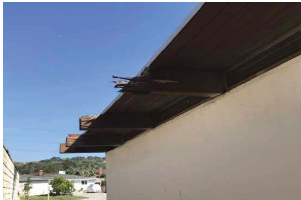
24 RESTROOM DAMAGED ROOF RAFTERS
