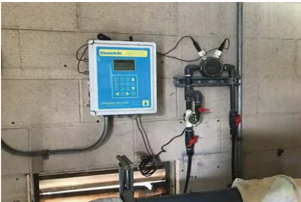
47 SWIMMING POOL CHEMICAL FEED SYSTEM
