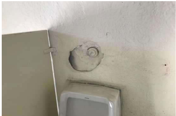
42 DAMAGED INTERIOR WALL FINISH
