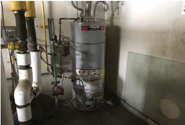
39 BUILDING 311 WATER HEATER
