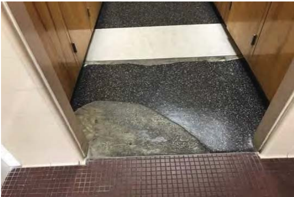
45 DAMAGED LOCKERS ROOM FLOOR
