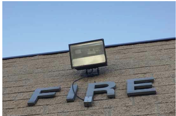
42 EXTERIOR BUILDING MOUNTED LIGHT
