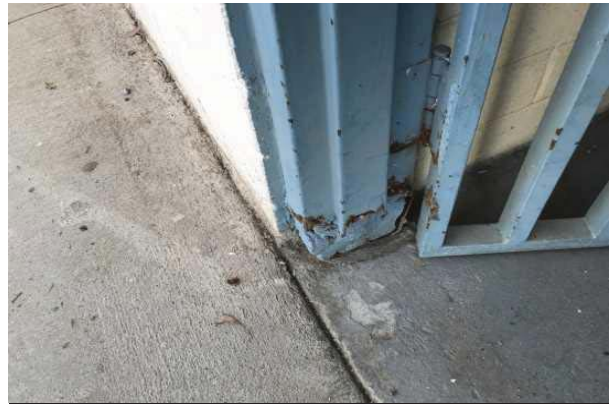
40 CORROSION AT EXTERIOR DOOR
