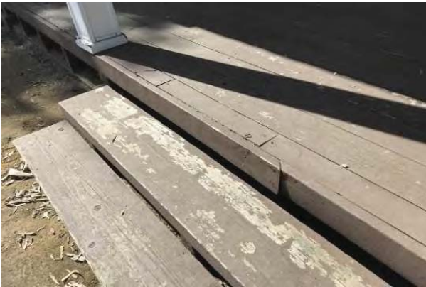
21 DAMAGED WOOD STAIRS
