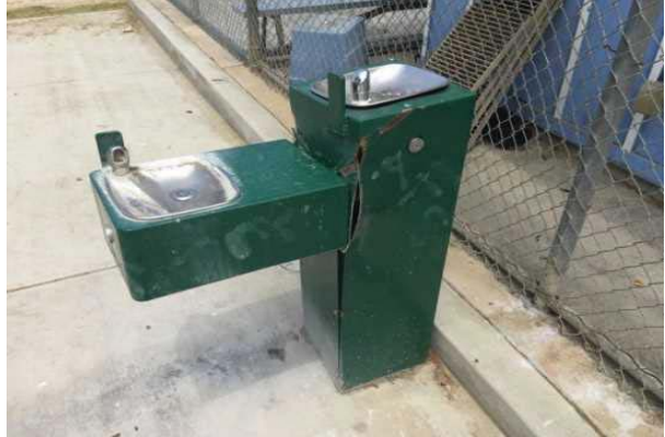
52 DAMAGED DRINKING FOUNTAIN
