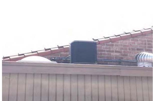
24 SPLIT-SYSTEM CONDENSING UNIT
