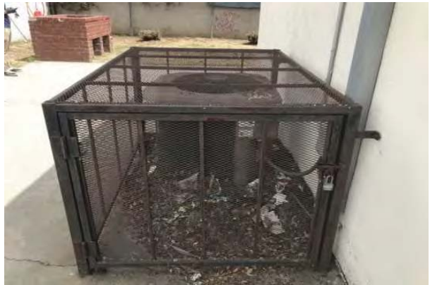
58 SCOUT HOUSE BUILDING CONDENSING UNIT
