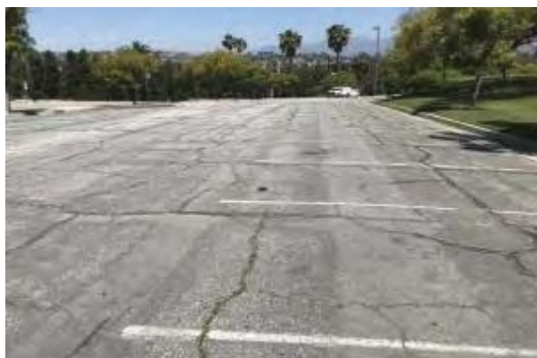
6 DETERIORATED PARKING LOTS
