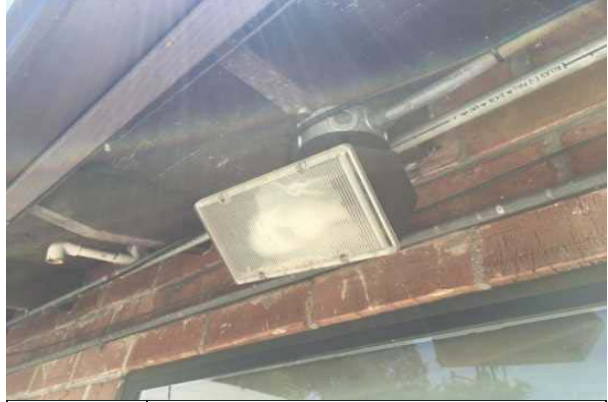
32 EXTERIOR BUILDING MOUNTED LIGHT
