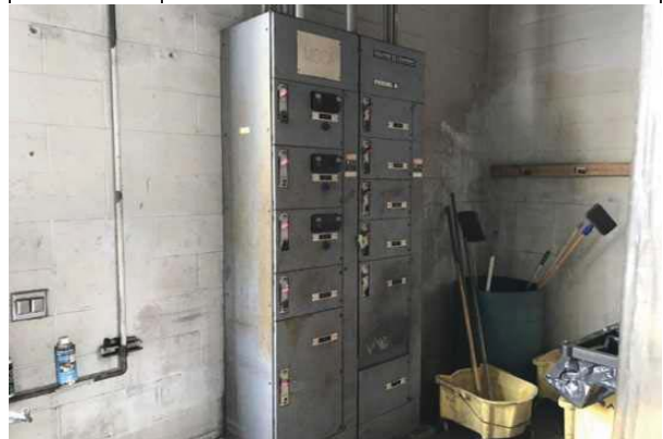
42 MOTOR CONTROL CENTER
