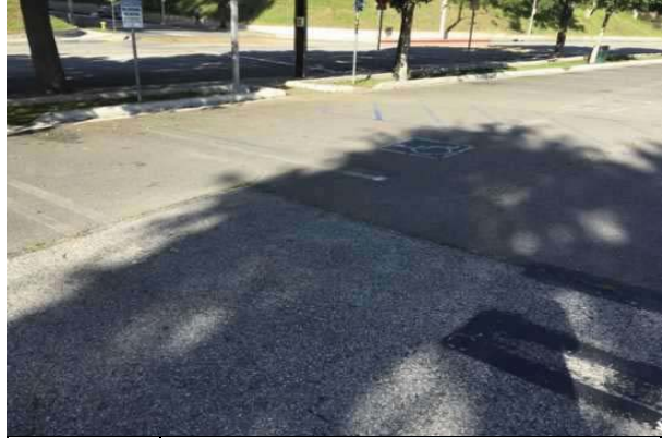
32 WORN ASPHALT PAVEMENT SEALING AND STRIPING
