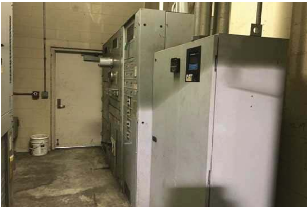
41 MAIN SWITCHBOARD (MAINTENANCE SHOP)
