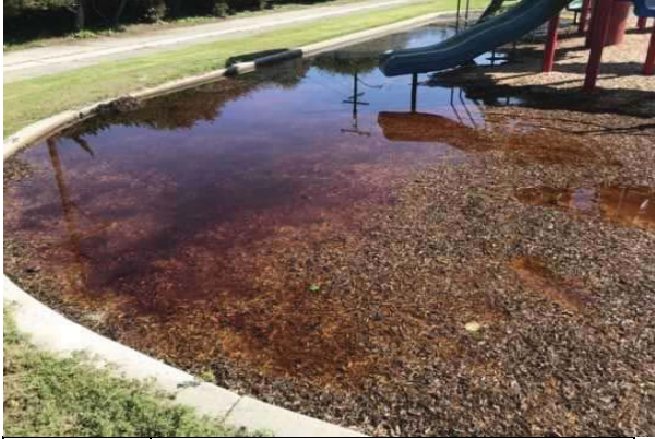
31 NORTH PLAYGROUND FLOODED AREA
