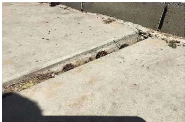
12 CONCRETE SIDEWALK TRIPPING HAZARD
