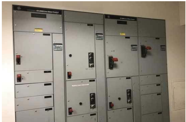
36 MOTOR CONTROL CENTER
