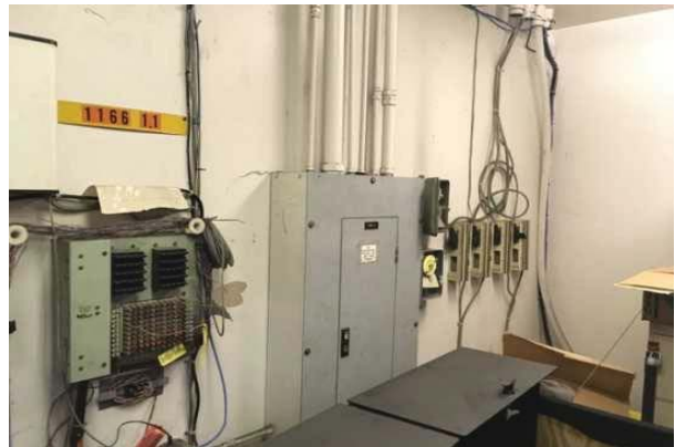
30 ELECTRICAL DISTRIBUTION SYSTEM
