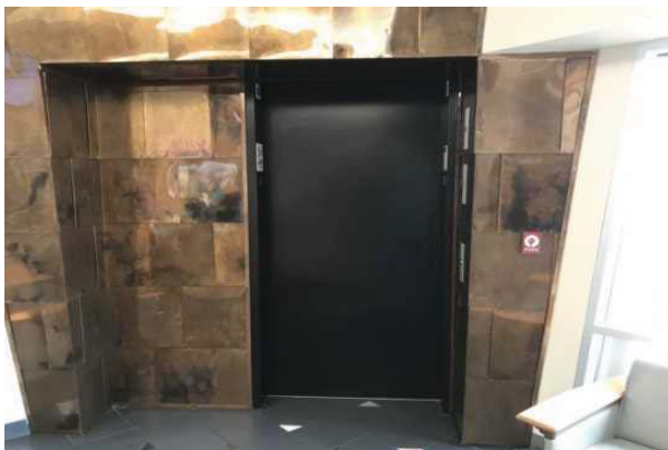
47 ELEVATOR CAB-MAIN OFFICE BUILDING
