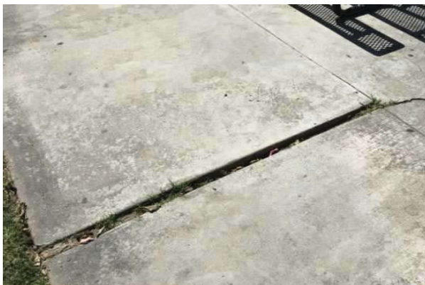
11 MISSING JOINT CAULKING IN CONCRETE SIDEWALK
