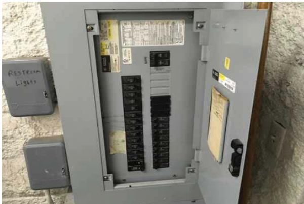
27 MAIN DISTRIBUTION PANEL
