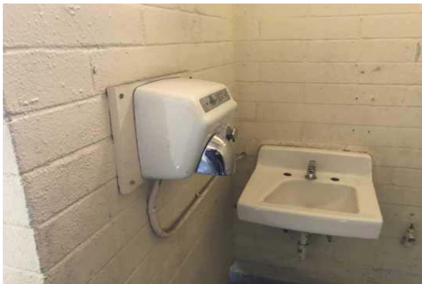
47 RESTROOM LAVATORY AND HAND DRYER
