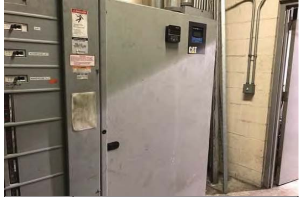
44 AUTOMATIC TRANSFER SWITCH (ATS)
