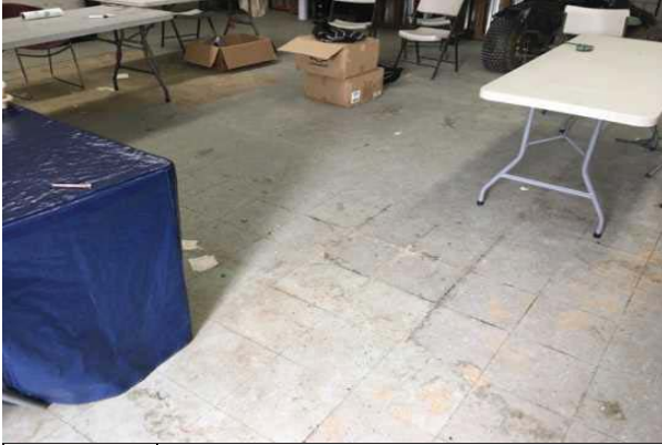
19 DAMAGED AND MISSING VCT
