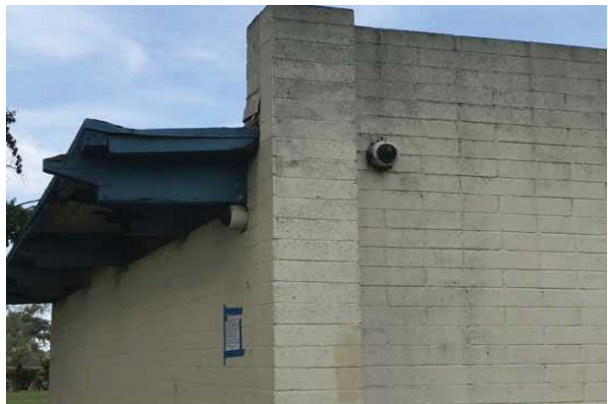
36 CAMERAS AND CCTV
