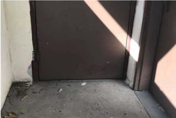
25 RESTROOM DAMAGED STUCCO
