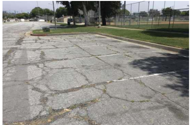
40 ASPHALT PAVEMENT WORN SEALING AND STRIPING
