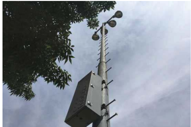
34 STADIUM POLE LIGHT
