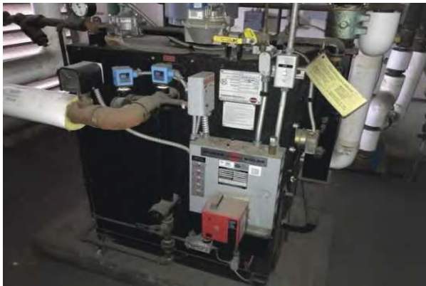
35 HVAC BOILER (BUILDING 311)
