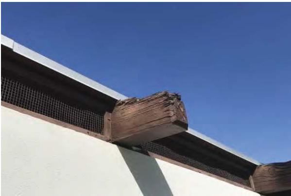
23 RESTROOM DAMAGED ROOF RAFTERS
