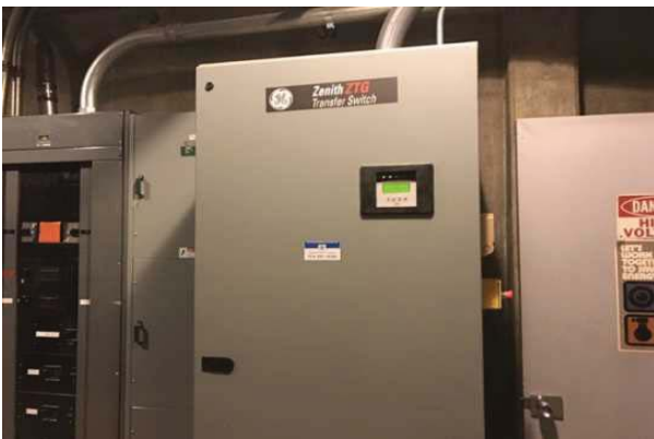
41 AUTOMATIC TRANSFER SWITCH
