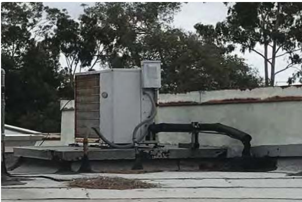
59 COMMUNITY CENTER SPLIT SYSTEM CONDENSER
